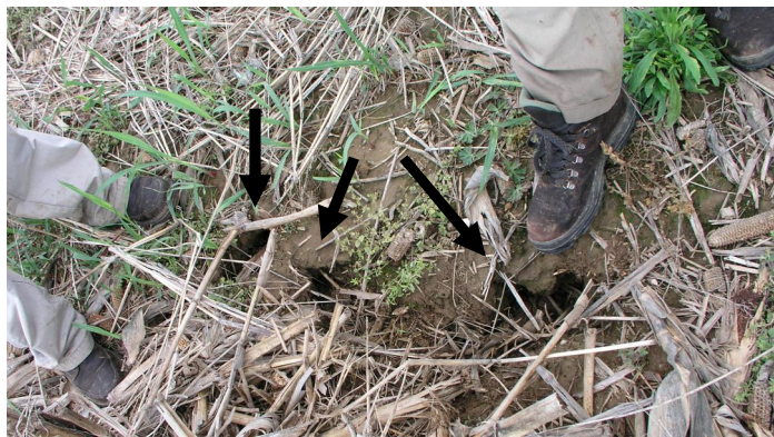
Figure 7. Photograph of epikarst swallow holes (indicated by arrows) along Linear 1 on the Newton farm.
